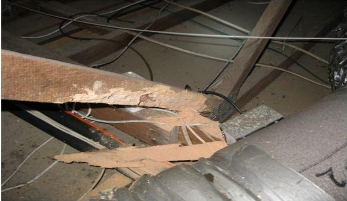
Figure 3. Lyctus attack on a truss member
