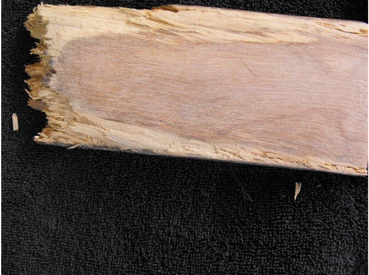
Figure 5. Decay in a blackbutt sapwood in a verandah joist
