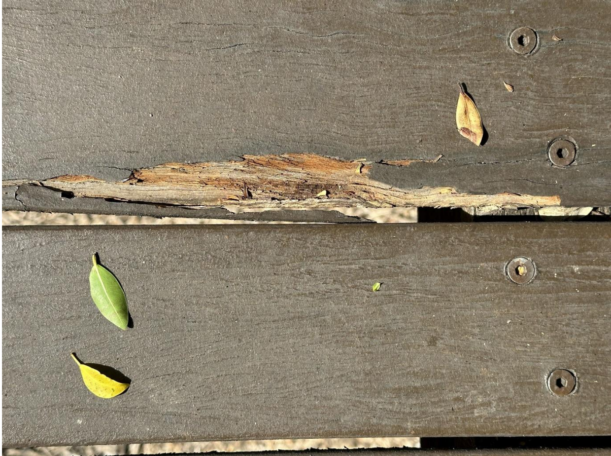
Figure 7. Untreated sapwood in sapwood is decaying
